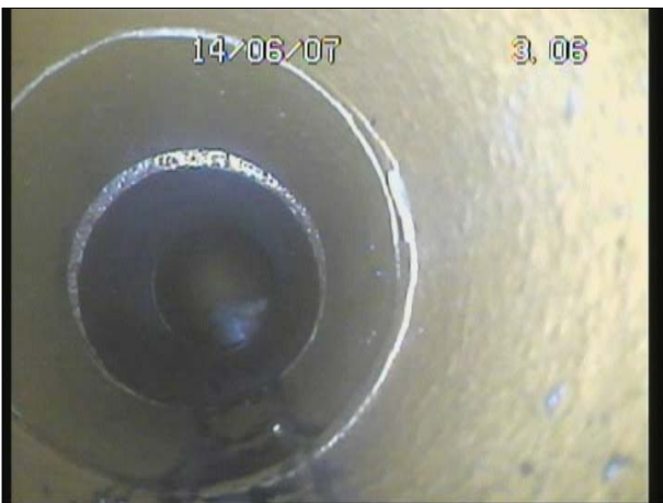
Photo: 12a, Tape No.: DVD, 00:00:00 3.06m, Circumferential Crack, from 12 to 12 o'clock
