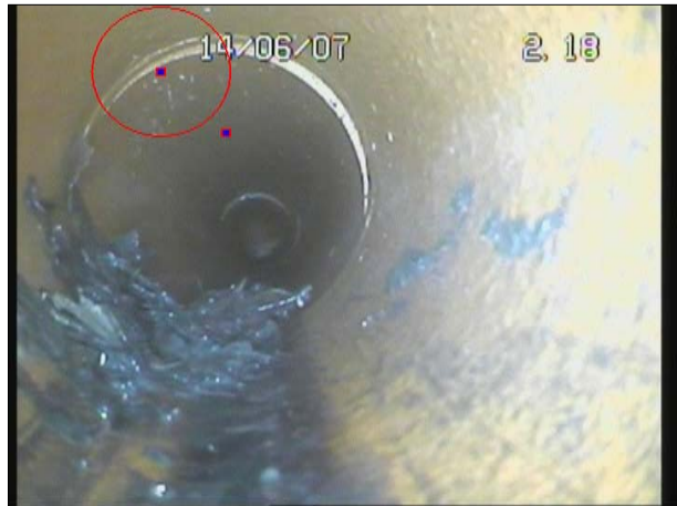
Photo: 1_4a, Tape No.: DVD, 00:00:00 2.18m, Circumferential Crack, from 09 to 03 o'clock
