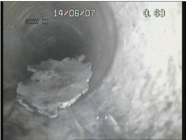
Photo: 2a, Tape No.: DVD, 00:00:00 0.2m, Debris, Start
