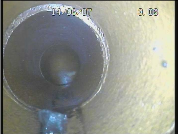
Photo: 6b, Tape No.: DVD, 00:00:00 3.1m, Joint displaced. Medium
