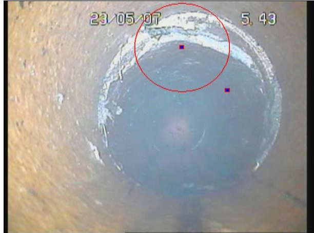
Photo: 1_10a, Tape No.: DVD, 00:00:00 5.5m, Open joint large
