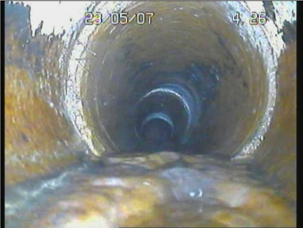
Photo: 9a, Tape No.: DVD, 00:00:00 4.3m, Joint displaced. Medium
