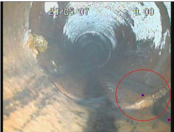
Photo: 1_6a, Tape No.: DVD, 00:00:00 3.1m, Joint displaced. Medium
