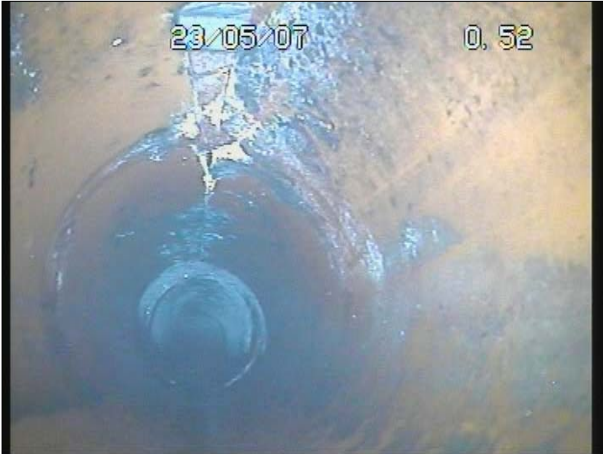
Photo: 3a, Tape No.: DVD, 00:00:00 0.5m, Longitudinal Crack, at 12 o'clock, Start
