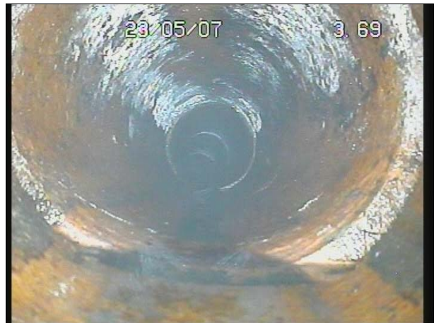
Photo: 8a, Tape No.: DVD, 00:00:00 3.7m, Joint displaced. Medium
