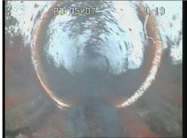
Photo: 4a, Tape No.: DVD, 00:00:00 1.2m, Joint displaced. Small
