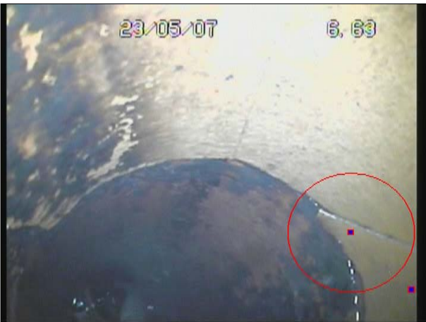
Photo: 1_13a, Tape No.: DVD, 00:00:00 6.6m, Longitudinal Crack, at 02 o'clock
