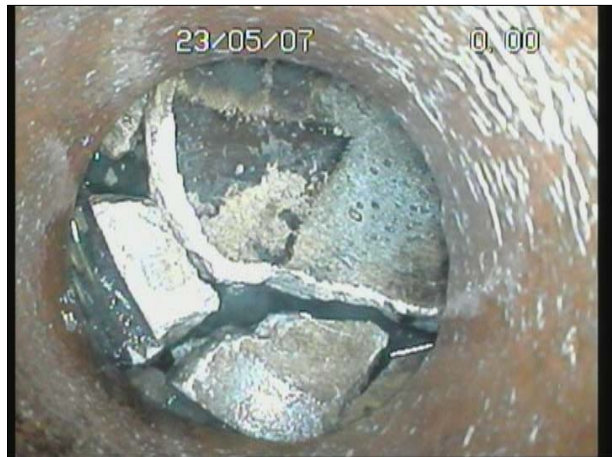
Photo: 2a, Tape No.: DVD, 00:00:00 7.1m, Broken Pipe - Base bend on tumbler before main sewer has broken
